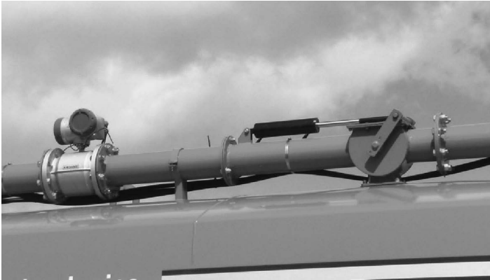
FIGURE 9.4 Flow meter and control valve.
