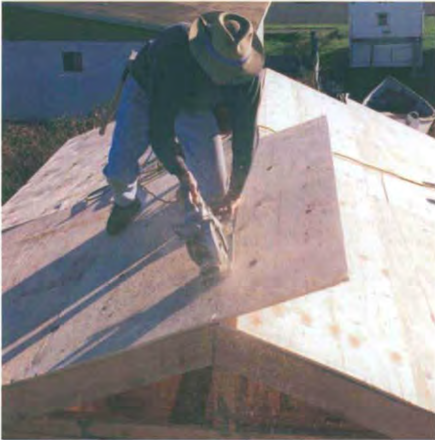
To cut the sheathing at the ridge on the roof, snap a chalkline along the ridge, set the saw to cut \frac{3}{4} in. deep, and make the cut. The sheathing doesn't have to fit perfectly here because it will be covered by paper and shingles. (Photo by Roe A. Osborn.)
