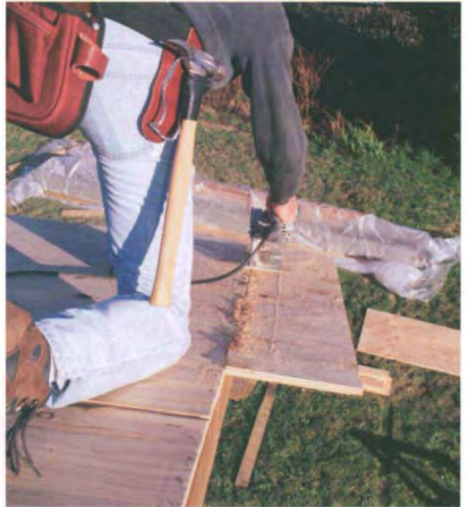
A last step in the roof-sheathing process is to trim the sheathing flush with the barge rafters at the gable ends. (Photo by Roe A. Osborn.)
