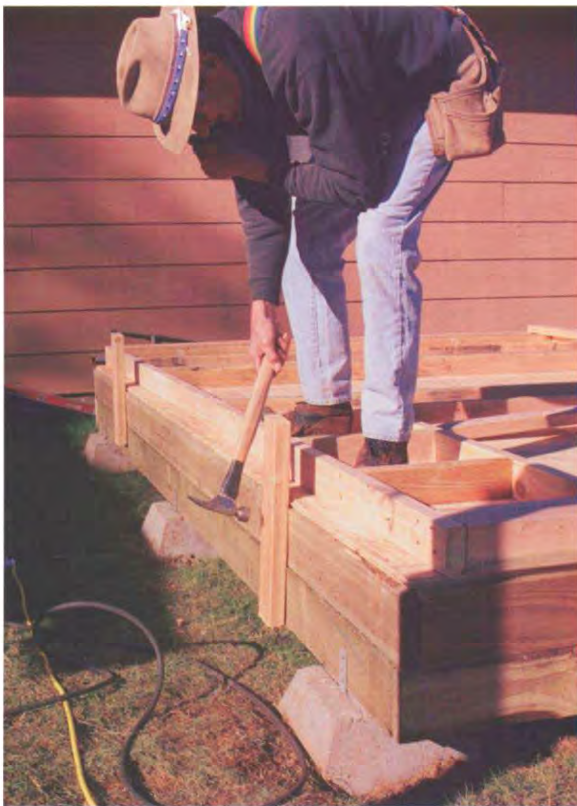
Nail lengths of 2x stock to the rim joist to keep an outside wall from slipping over the edge when it is raised. (Photo by Roe A. Osborn.)
