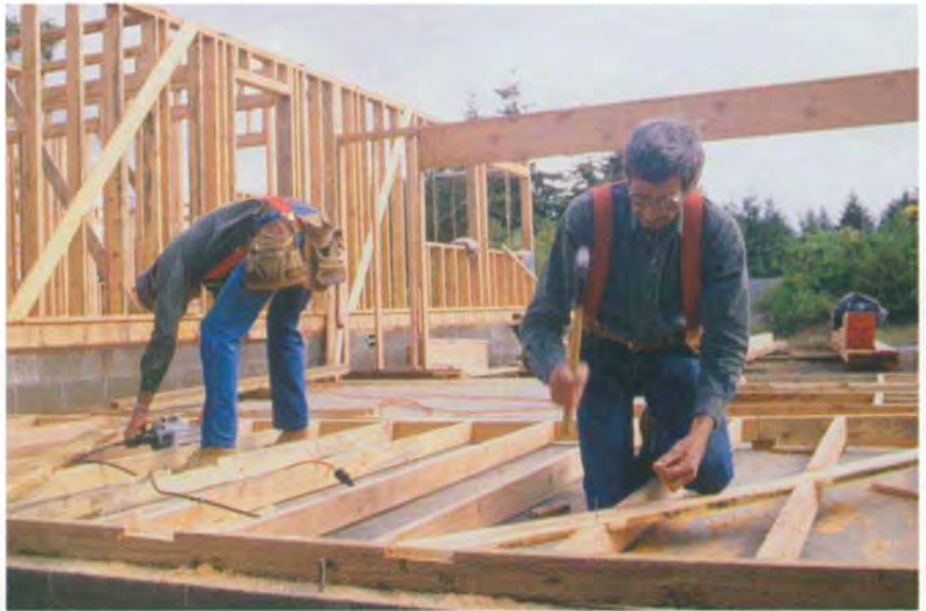
Studs are the vertical members that make up the frame of a wall and usually are spaced 16 in. o.c. or 24 in. o.c. (Photo by Roger Turk.)
