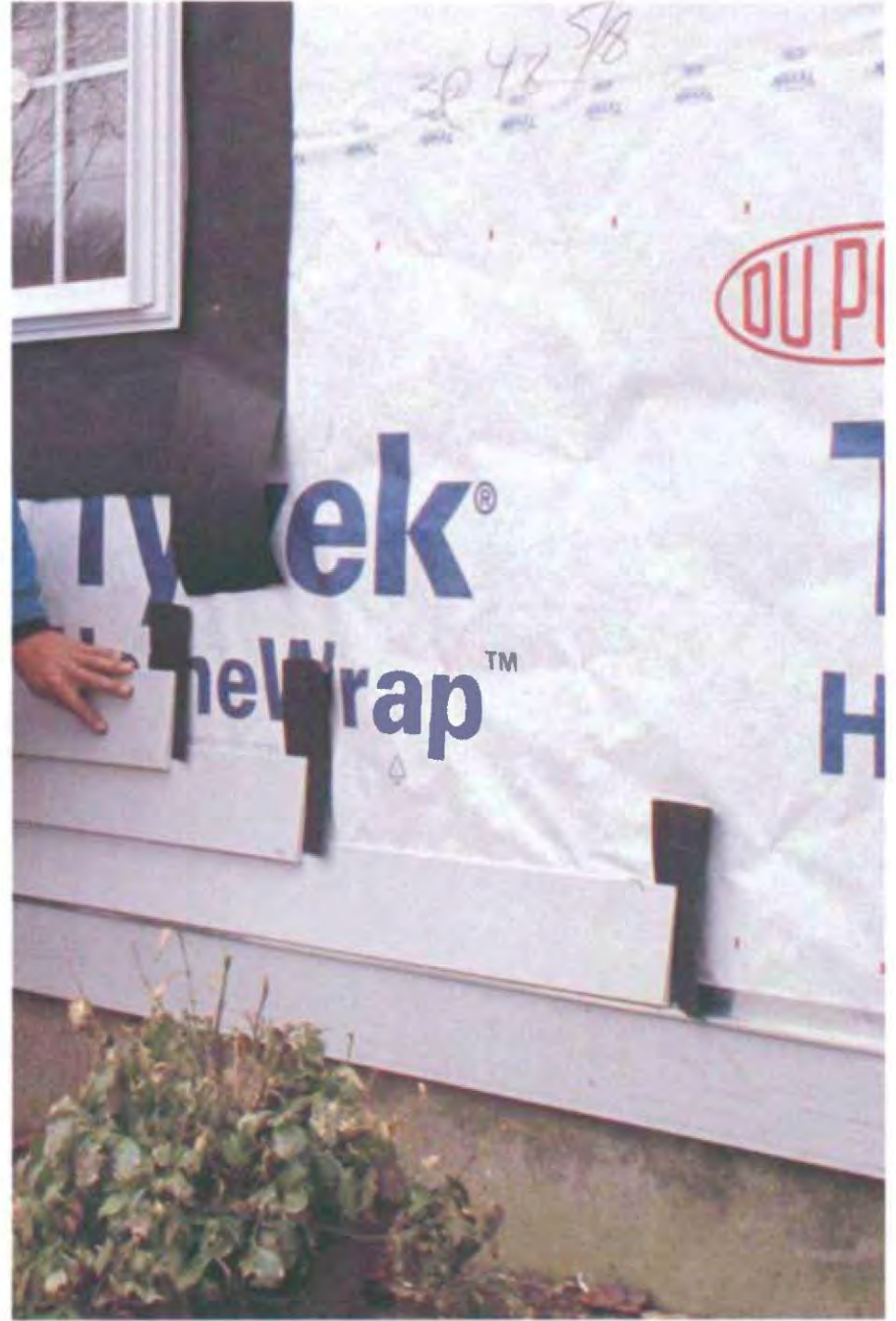
Where a great deal of rain is likely, it's a good idea to tack 4-in. by 12-in. felt strips behind all butt joints on horizontal siding. These strips provide extra protection against moisture intrusion. (Photo by Andrew Engel.)
