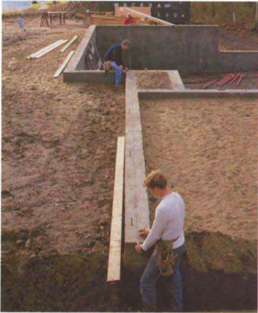
A house foundation can be a combination of full concrete basement and concrete stemwalls enclosing a crawl space, such as shown here, or just stemwalls with a crawl space, a concrete slab, or concrete piers on footings. (Photo by Roe A. Osborn.)
