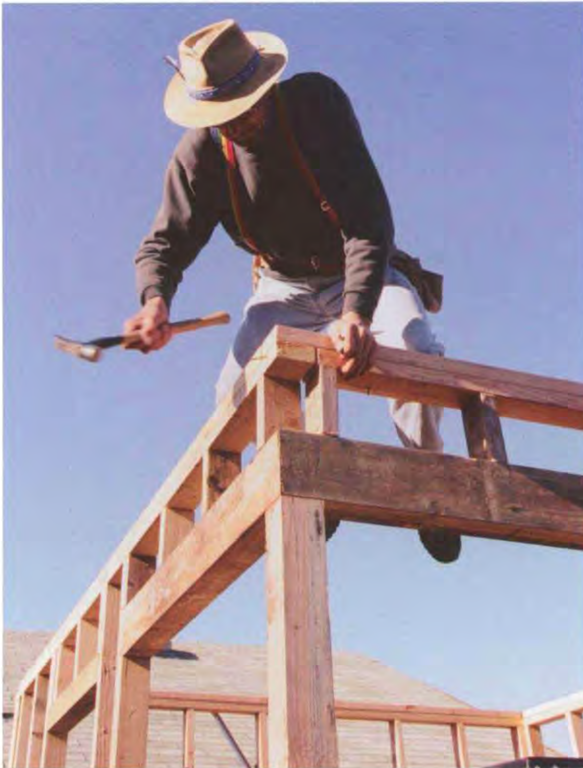
Carpenters use 16d nails for most rough framing, such as nailing top plates together. (Photo by Roe A. Osborn.)
