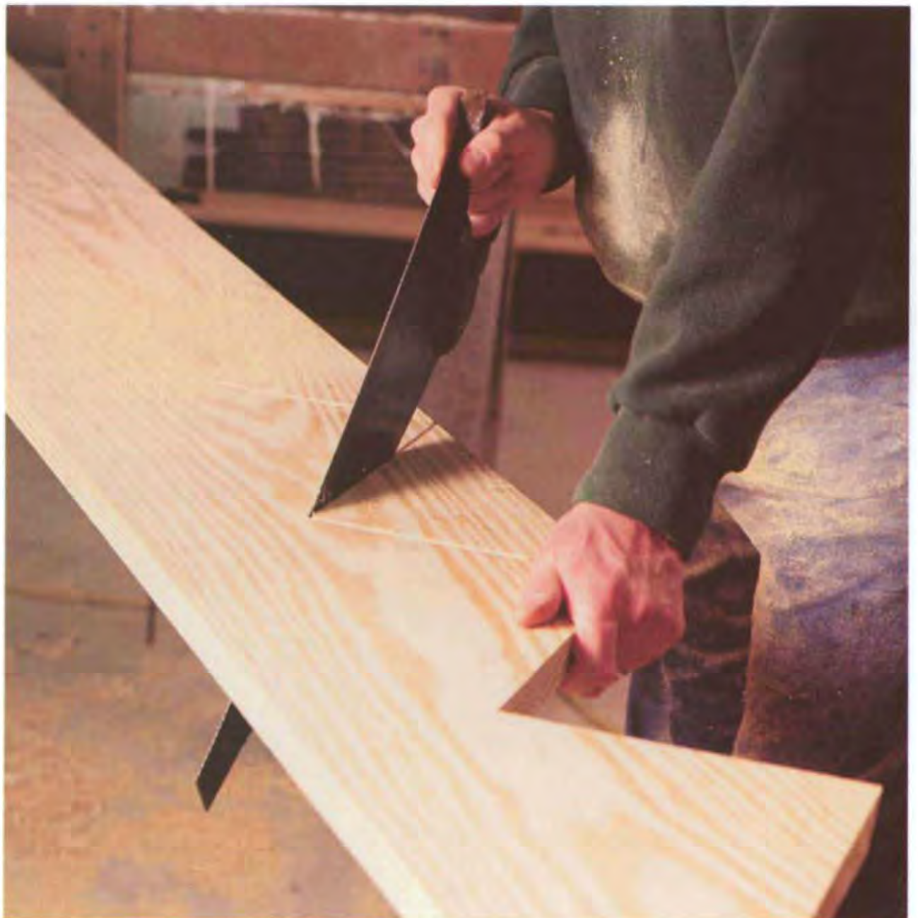
The notch in the rough stringers can be overcut with a circular saw. If the stringers are exposed, finish the cut with a handsaw or jigsaw. (Photo by Scott Phillips.)
