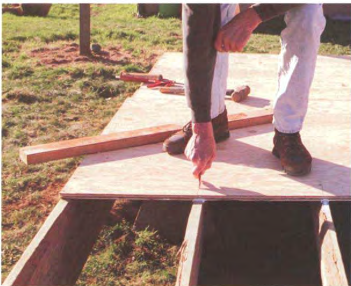
After each row of sheathing has been installed, mark the joist location on top at the leading edge so you will know where to drive the nails. (Photo by Roe A. Osborn.)
