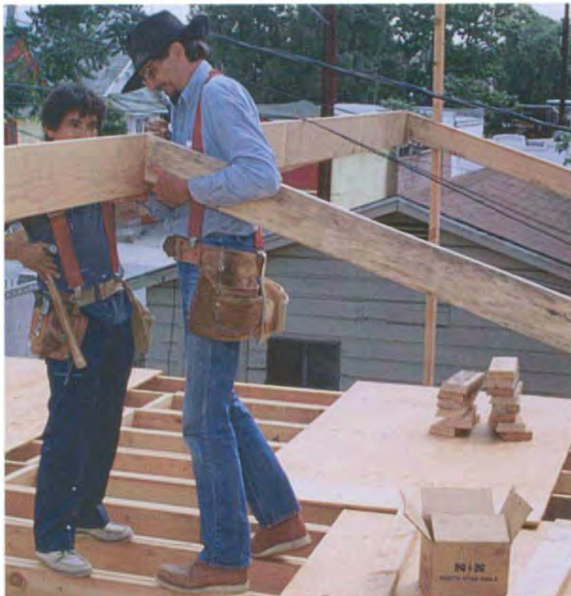
Toenail a pair of rafters to the top plates, then raise the ridge board between the rafters. Nail the rafters to the ridge board with 16d nails. (Photo by Robert Wedemeyer.)
