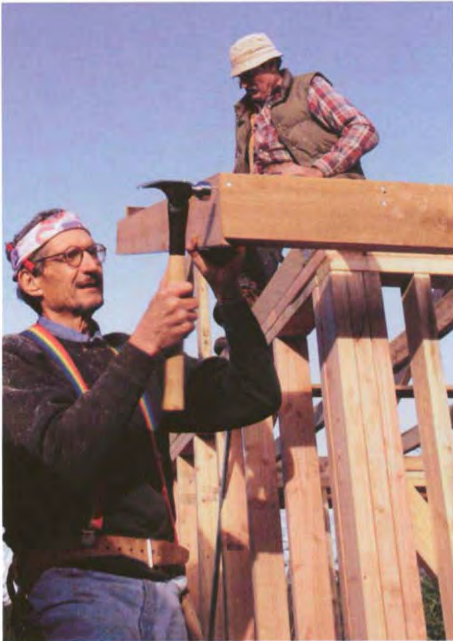
Drive two 16d hot-dipped galvanized nails through the barge rafter and into the fascia. Make sure the miter joint is tight because it will be seen. (Photo by Roe A. Osborn.)
