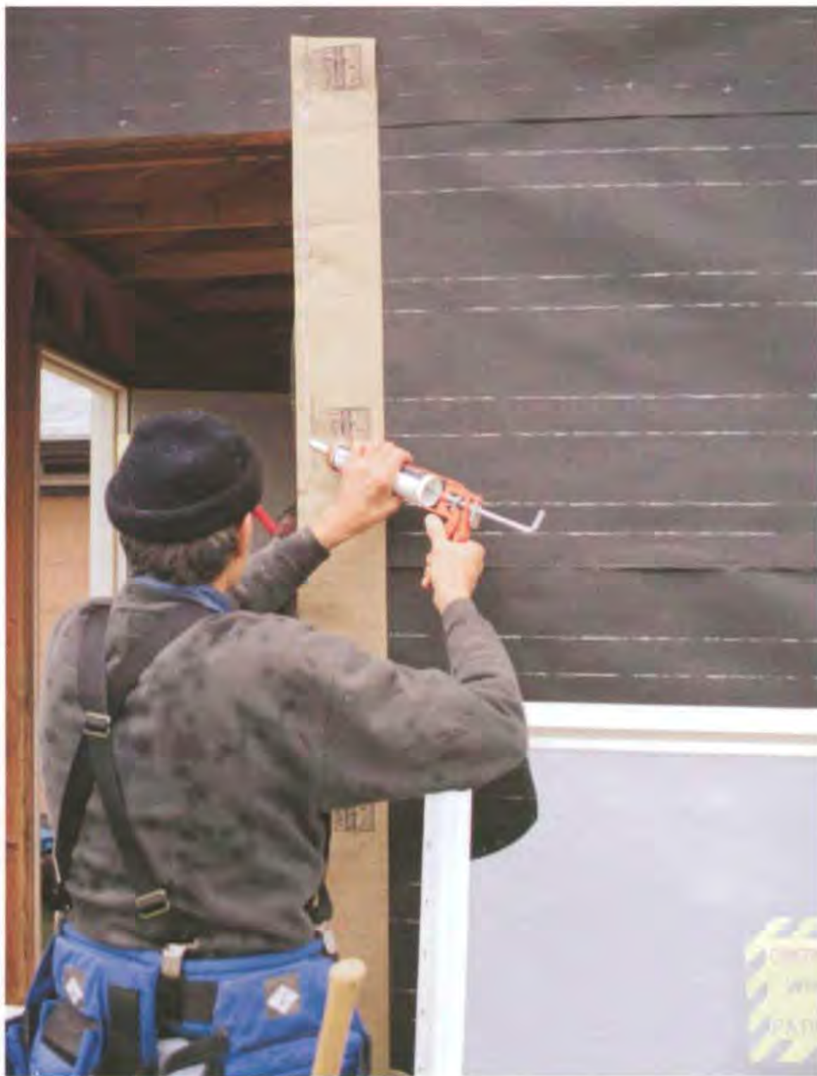
Before nailing the window in place, lay down a good bead of silicone caulk around the entire opening under the window flange. This helps keep water from entering around the window frame. (Photo by Roe A. Osborn.)
