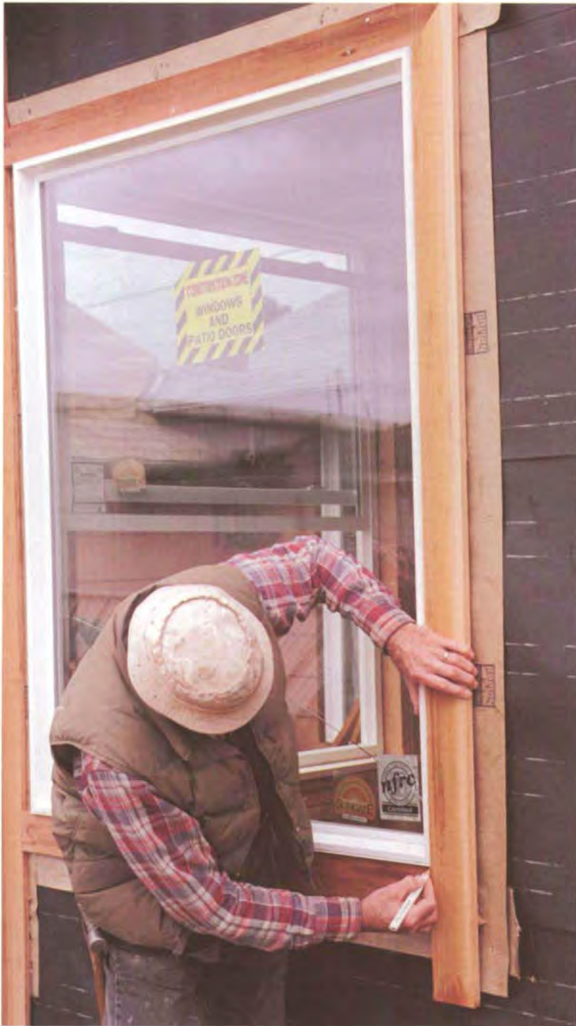
After fitting the miter joint at the top, scribe the miter on the bottom. Mark the miter cut at the window corner and make the cut. (Photo by Roe A. Osborn.)
