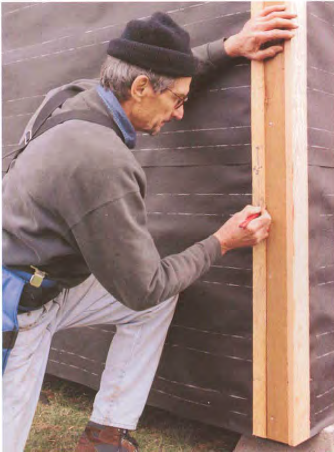
Transfer the marks on the story pole to each piece of vertical house trim. The marks will ensure that the siding will be the same height on all sides of the house. (Photo by Roe A. Osborn.)
