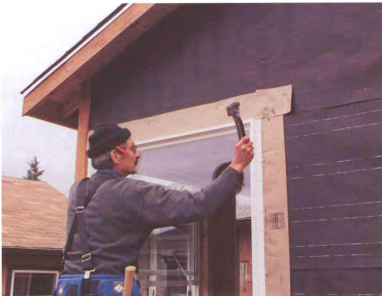
After nailing the window in place, run another bead of caulk at the top of the flange, then staple the last strip of felt paper. (Photo by Roe A. Osborn.)
