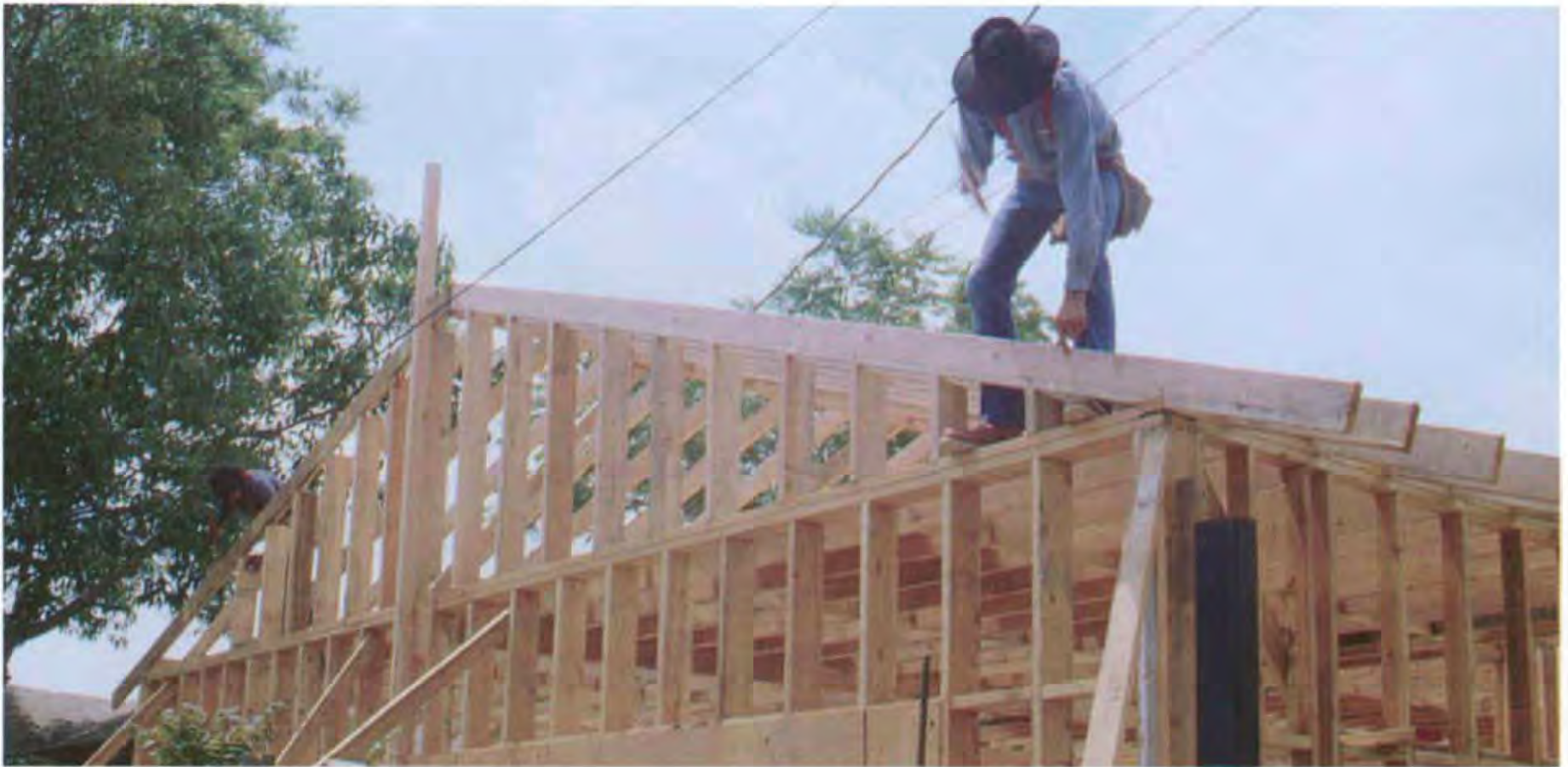
Be sure to nail the gable-end studs in plumb, trusting your eye or using a level. (Photo by Robert Wedemeyer.)
