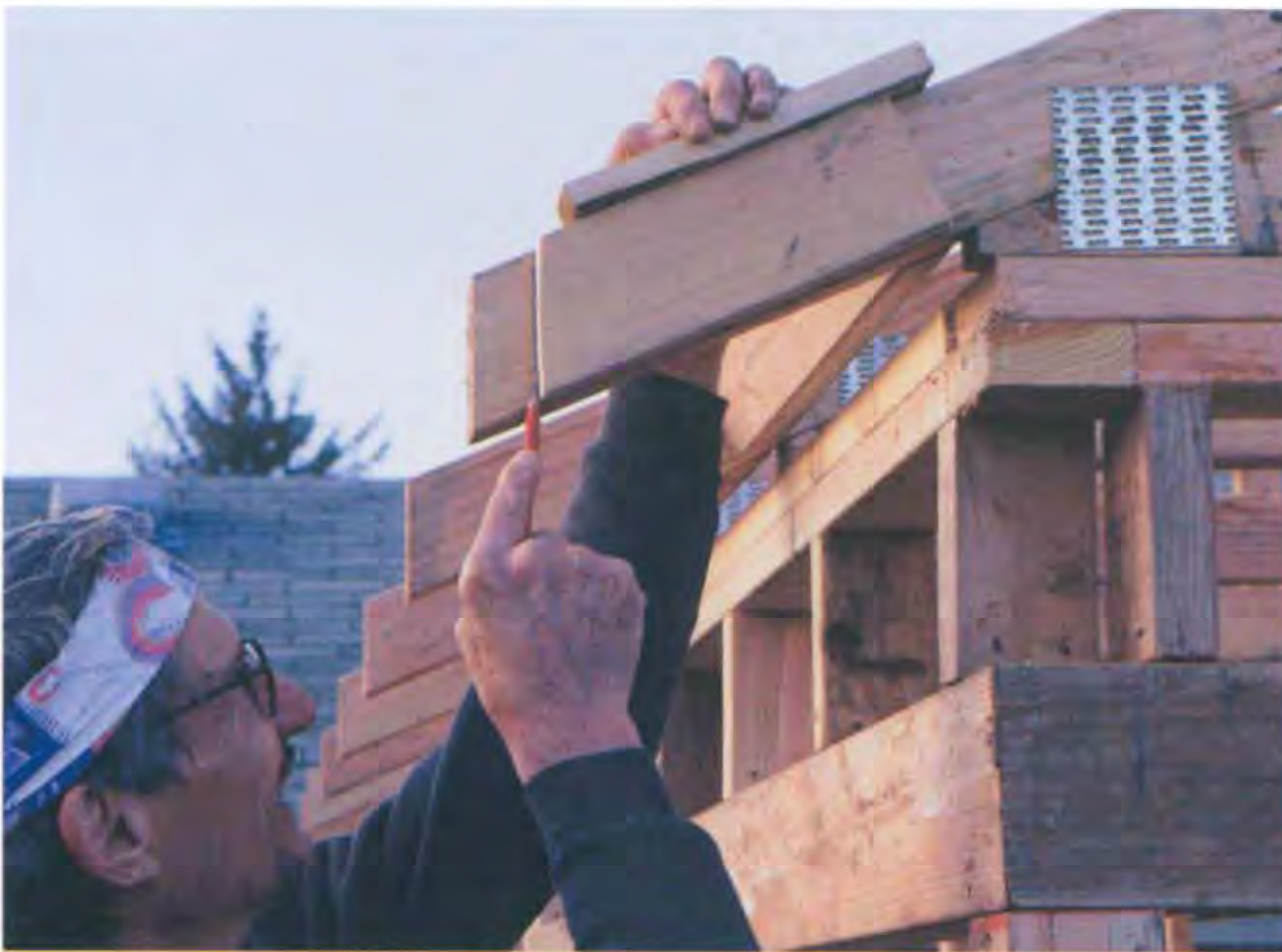
Place the fence of the rafter-cutting template on each rafter and scribe a plumb-cut line at the mark. (Photo by Roe A. Osborn.)
