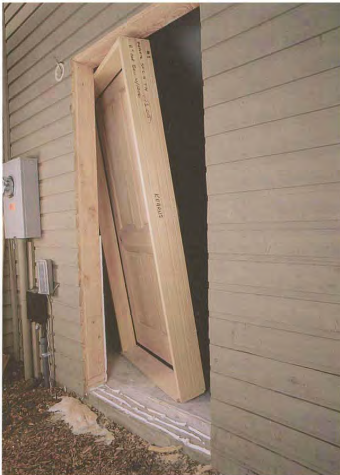
Part of the job of installing a prehung door is to lay a good-sized bead of silicone caulk under the door sill and around the opening under the factory-applied trim. (Photo by Charles Miller.)
