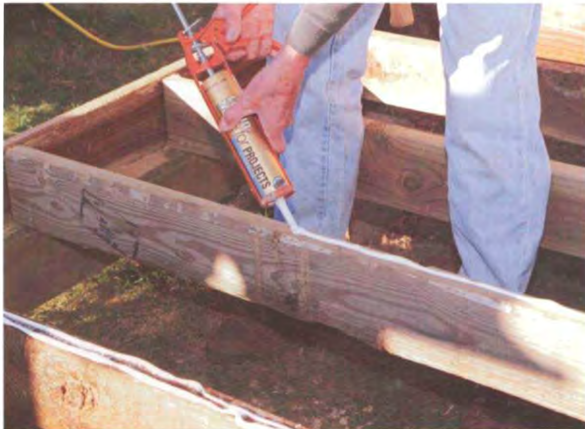
Construction adhesive helps secure sheathing tight to the joists and reduce floor squeaks. Place a \frac{1}{4} -in. bead on each joist. (Photo by Roe A. Osborn.)
