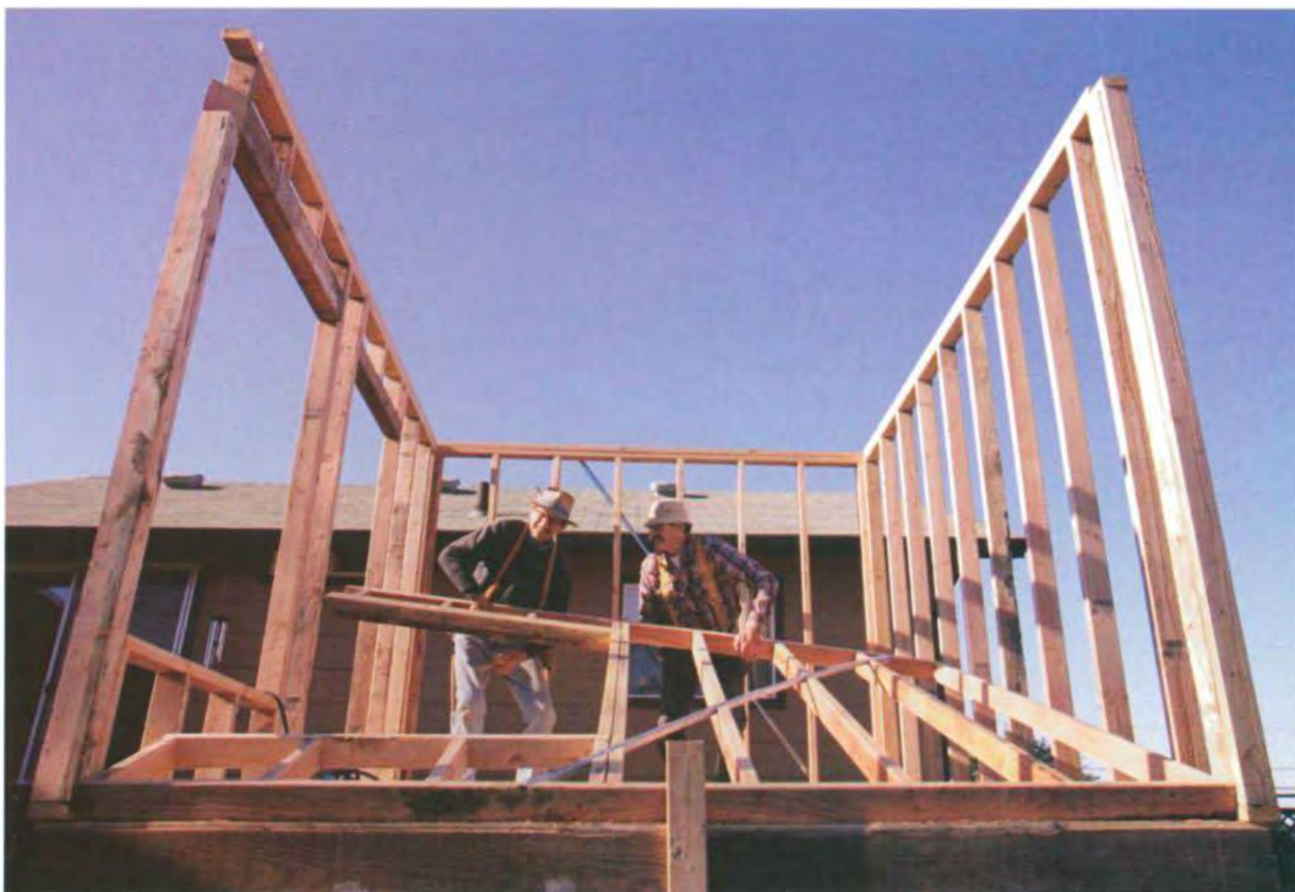
After the first wall is done, nail together another outside through wall, raise it, and brace it. Then build and raise the butt walls. (Photo by Roe A. Osborn.)
