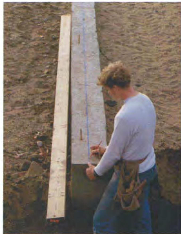
Chalklines on top of the concrete foundation indicate the position of the sill plates. (Photo by Roe A. Osborn.)
