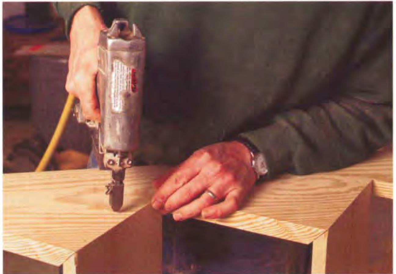
Before nailing on the treads, first nail on the risers, driving two 8d nails through the stringer into each riser board. (Photo by Scott Phillips.)
