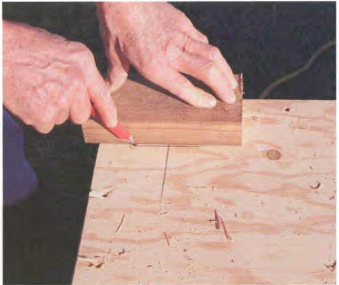
To lay out the wall locations at a corner, place a 2x4 or 2x6 block flush with the outside of the building and mark on the inside with a pencil. (Photo by Roe A. Osborn.)
