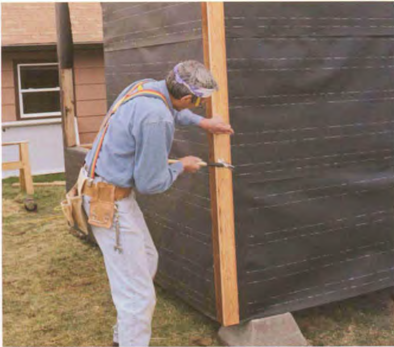
At the corners, I often nail a 1x3 on one side and install a 1x4 on the opposite side so that it laps the 1x3. Once lapped, both trim pieces look like a 1x4. (Photo by Roe A. Osborn.)
