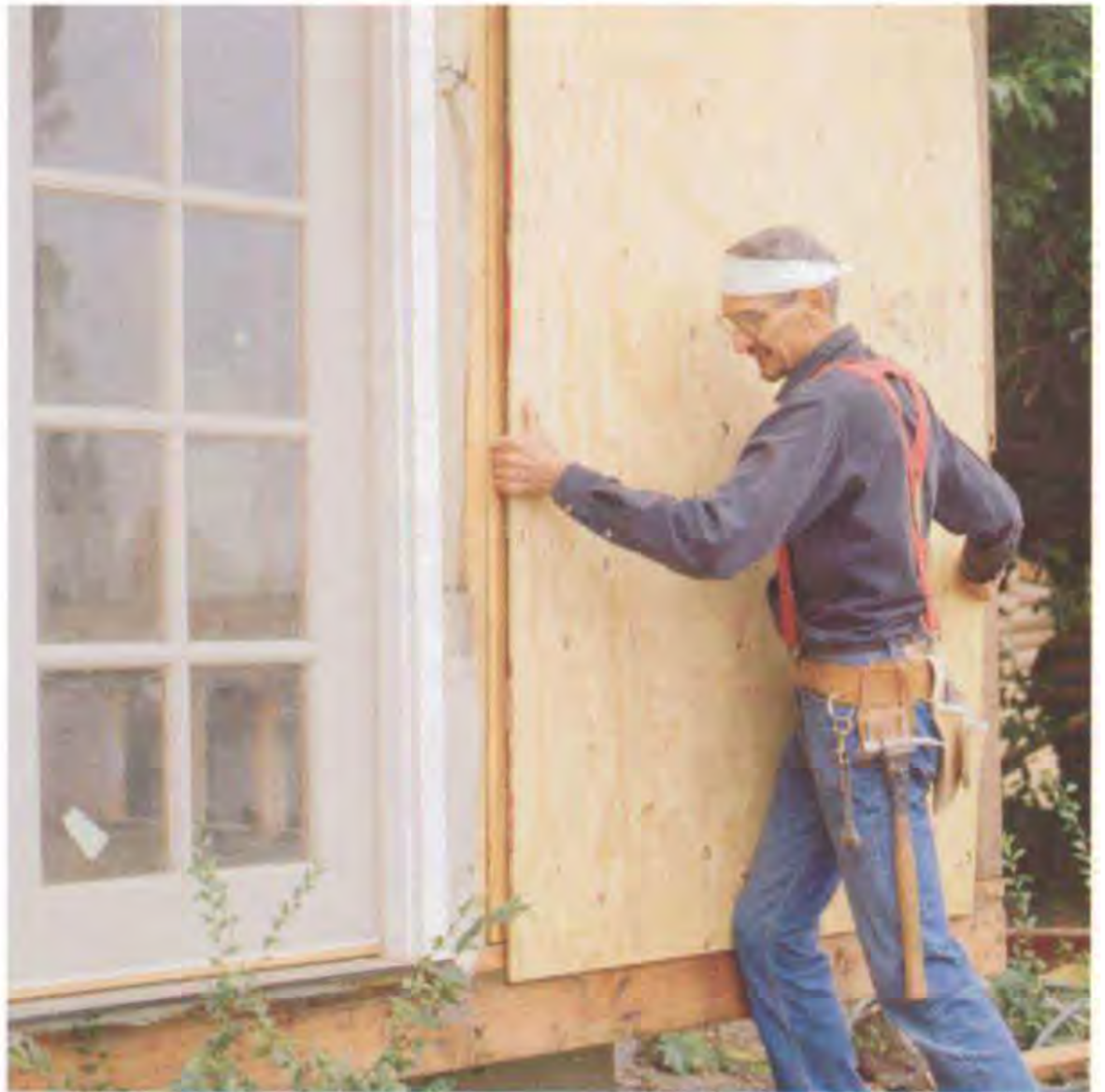
In most areas, codes allow wall sheathing to be installed vertically, with the long edges nailed to the wall studs. (Photo by Joe Haun.)
