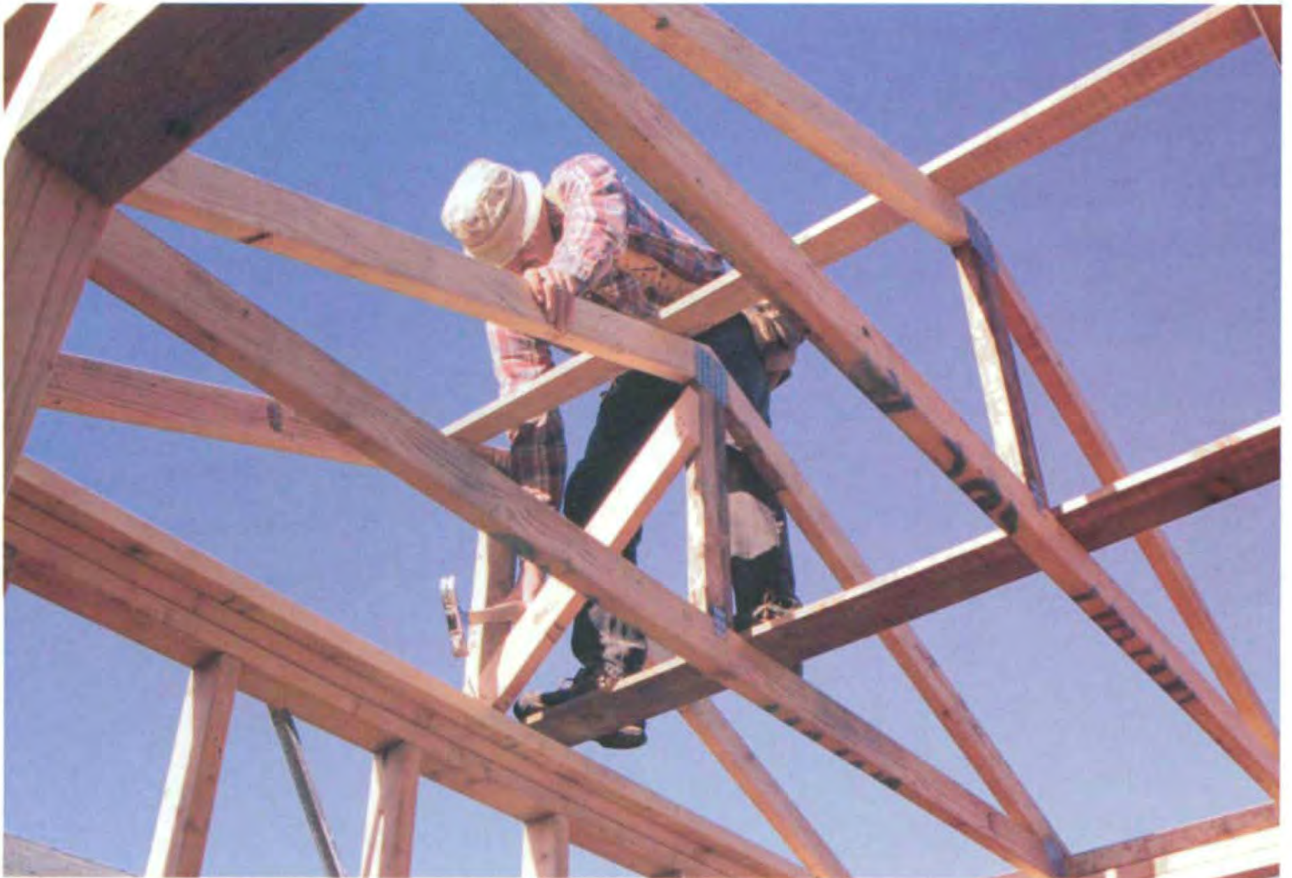
Sway braces at the gable ends and a catwalk on the joist chords help brace the roof. The 1x6 along the top of the rafters helps maintain the truss spacing until the sheathing is installed. (Photo by Roe A. Osborn.)
