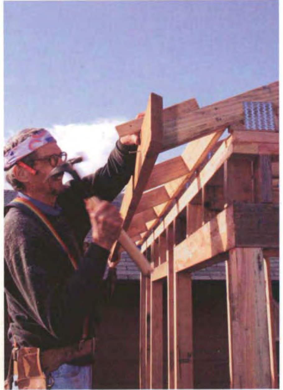
Place a piece of scrap wood on the top edge of a rafter extending beyond the rafter tail. Put the fascia snug against this scrap and drive one 16d galvanized nail high and another low. (Photo by Roe A. Osborn.)
