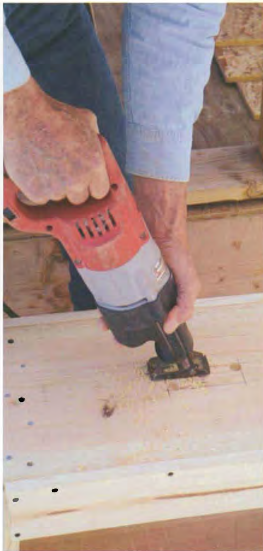
Cut out the handhold using a reciprocating saw (as shown) or a jigsaw.
