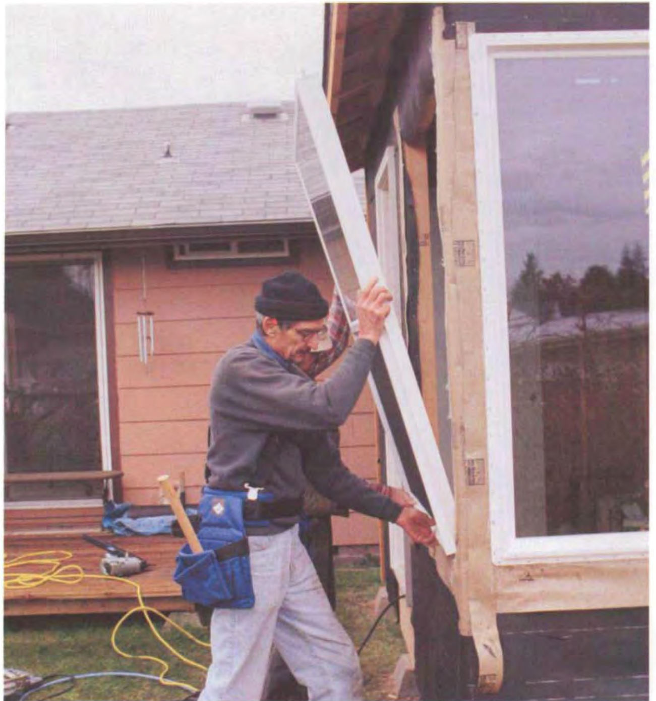
If the framing is correct, a window should fit easily in its rough opening. (Photo by Roe A. Osborn.)
