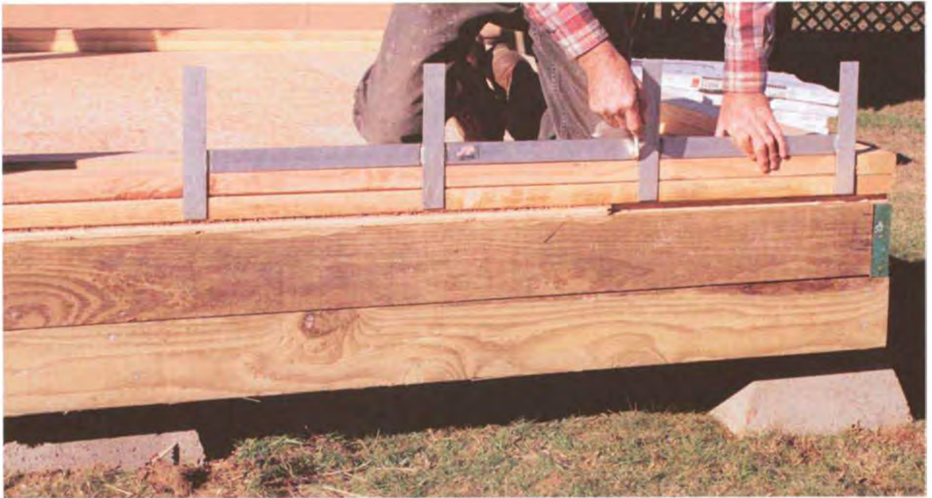
Use a layout stick to mark stud locations on wall plates. (Photo by Roe A.Osborn.)
