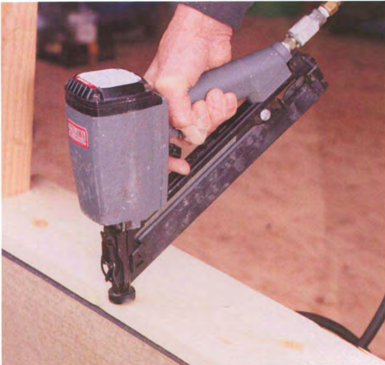
A finish nailer works well for trimwork, such as nailing in the stool for a window. (Photo by Roe A. Osborn.)
