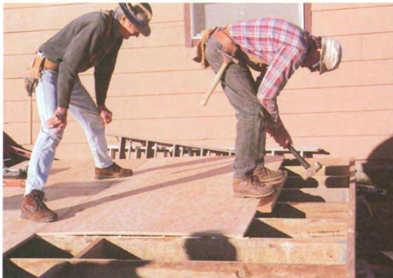
Sometimes T&G plywood needs some not-so-gentle persuasion. Have one person stand on the sheet to hold it flat and snug against the previous row while another hits it with a sledgehammer. The 2x placed in front of the sheet protects the plywood edge from damage. (Photo by Roe A. Osborn.)
