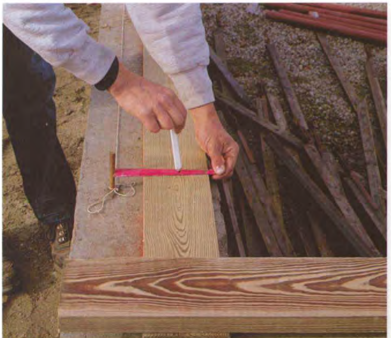
A simple measuring device called a bolt marker can be used to locate the bolt holes. With the sill plate lined up on the inside of the chalkline, hold the end of the marker against the bolt and mark the bolt hole. (Photo by Roe A. Osborn.)
