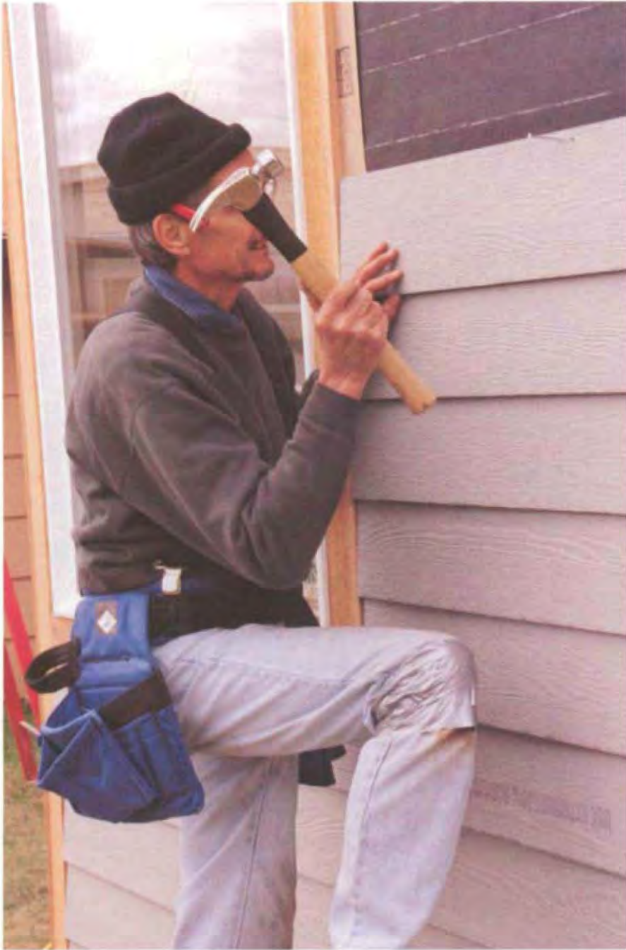
Once the siding begins going up, the house acquires a more finished look. However, it's important that siding be primed on all sides, including the back and especially the cut ends to prevent moisture problems. (Photo by Roe A. Osborn.)
