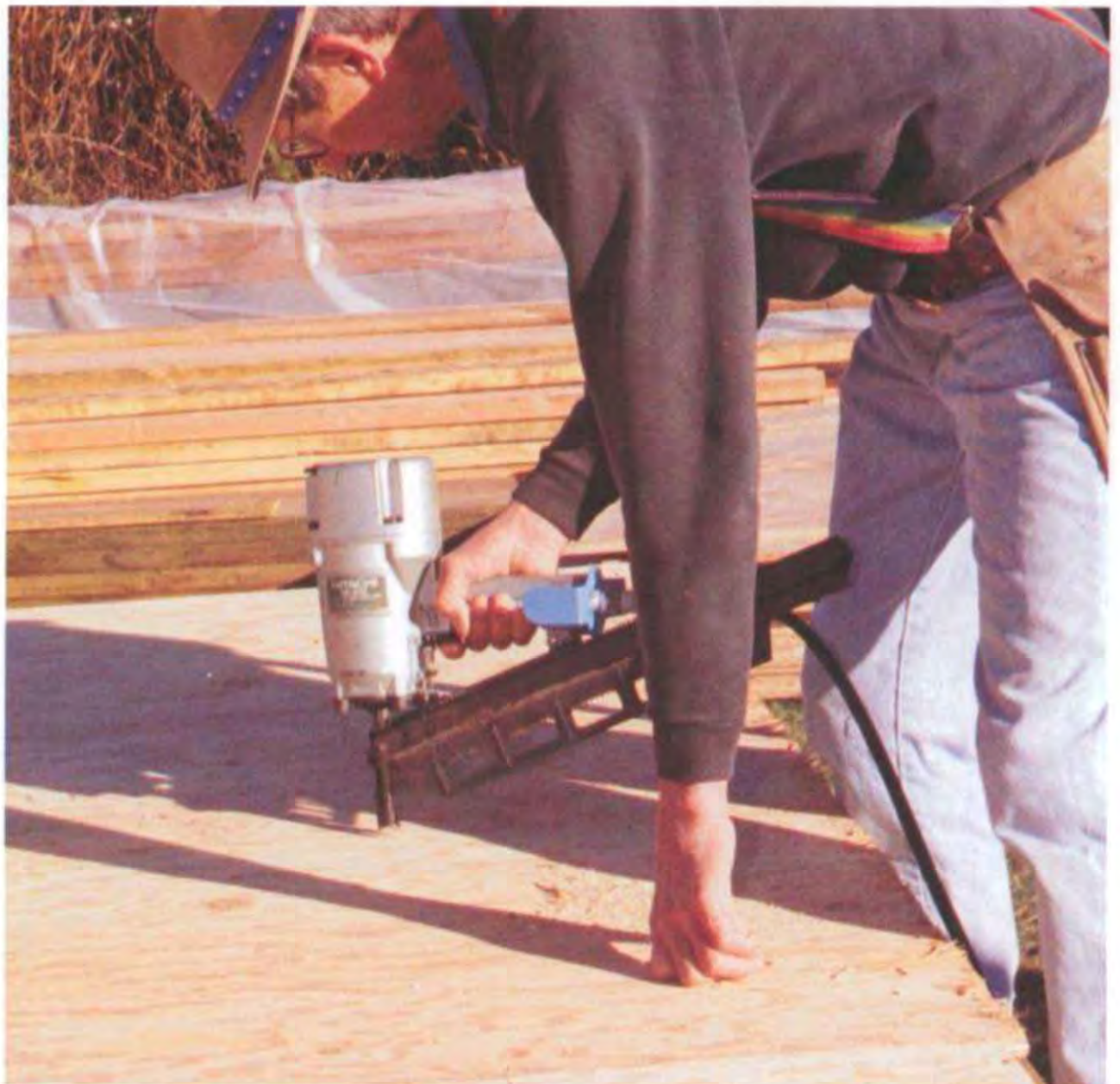
A framing nailer can be used for rough framing, as well as for nailing a plywood subfloor to joists. (Photo by Roe A. Osborn.)
