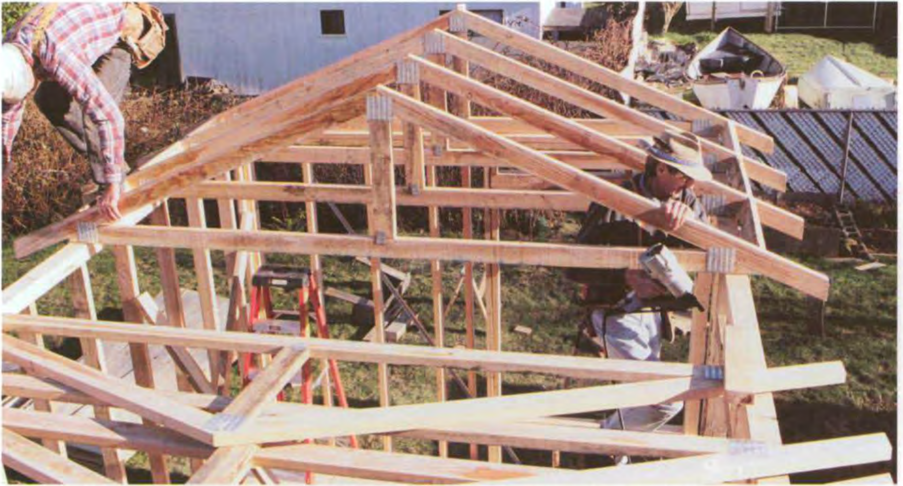
Roof trusses, which are delivered to the site fully assembled, simplify roof construction. Notice the frieze blocks (on right) between these king-post trusses, which help tie the whole roof together. (Photo by Roe A. Osborn.)
