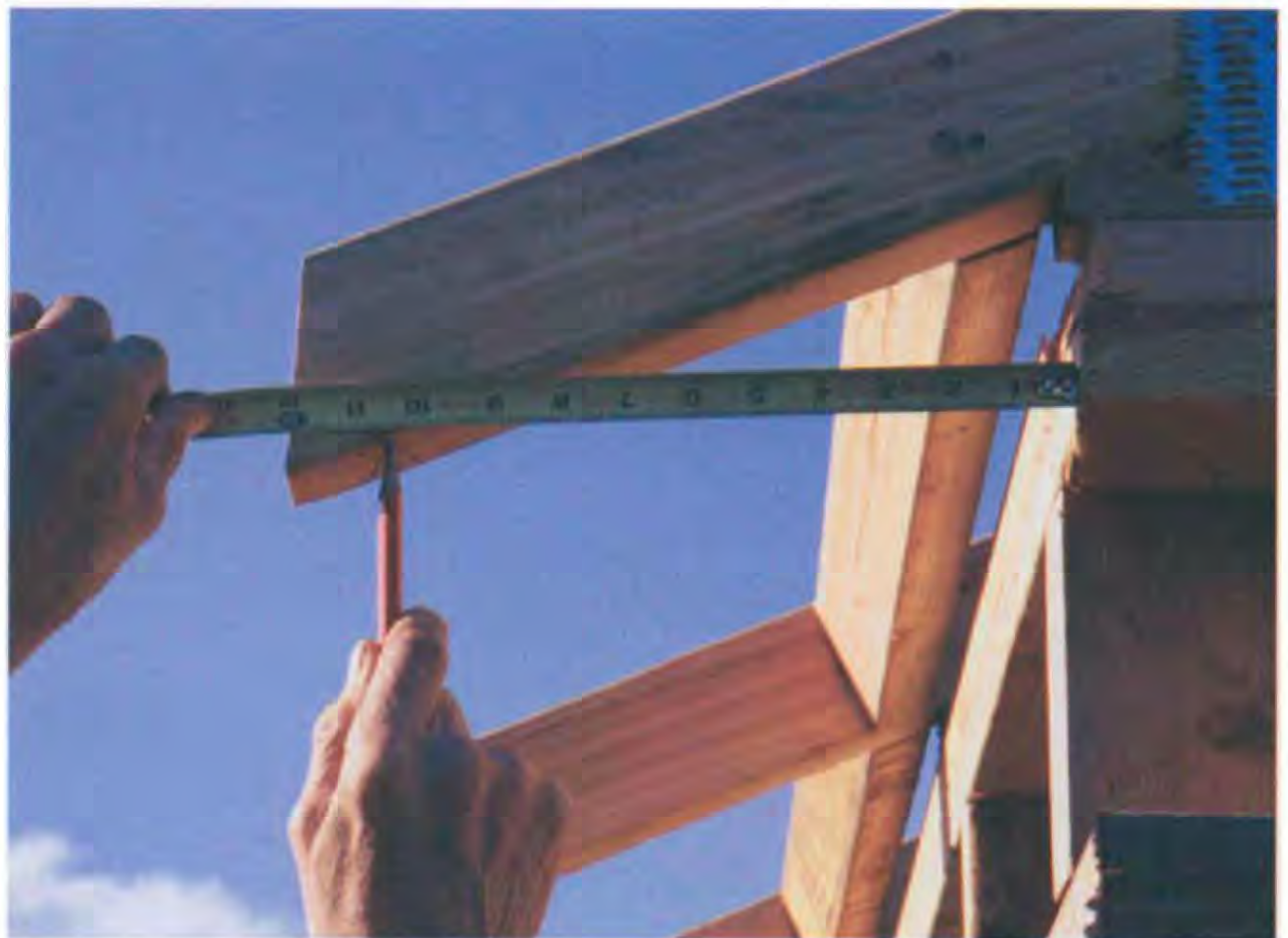
Measure straight out from the building on the gable-end rafters 10½ in. and make a mark. This will be the cut line. (Photo by Roe A. Osborn.)
