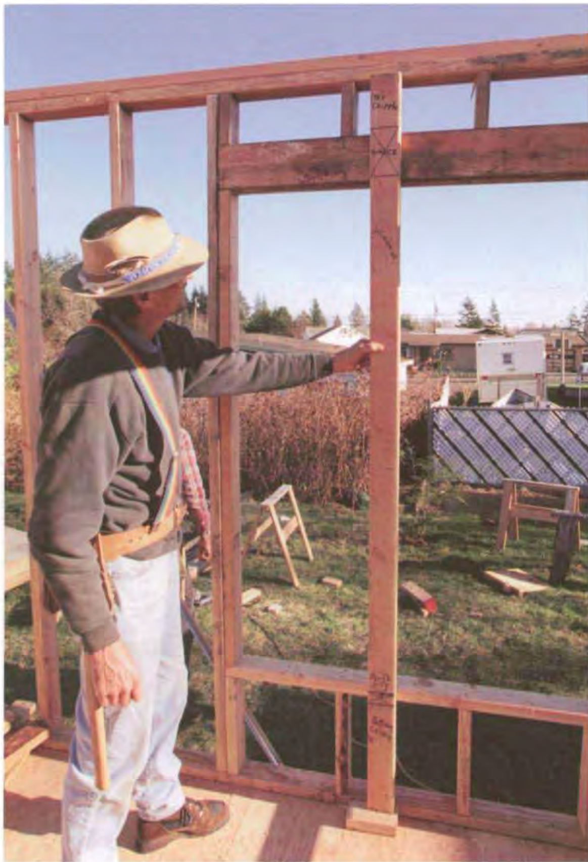
A story pole shows locations of headers and sills and the lengths of cripples and trimmers. (Photo by Roe A. Osborn.)
