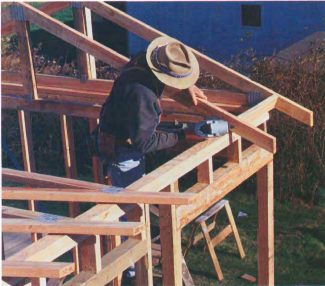
Toenail the joist chord to the top plate with two 16d nails, then drive two more through the rafter chord into the frieze block. (Photo by Roe A. Osborn.)
