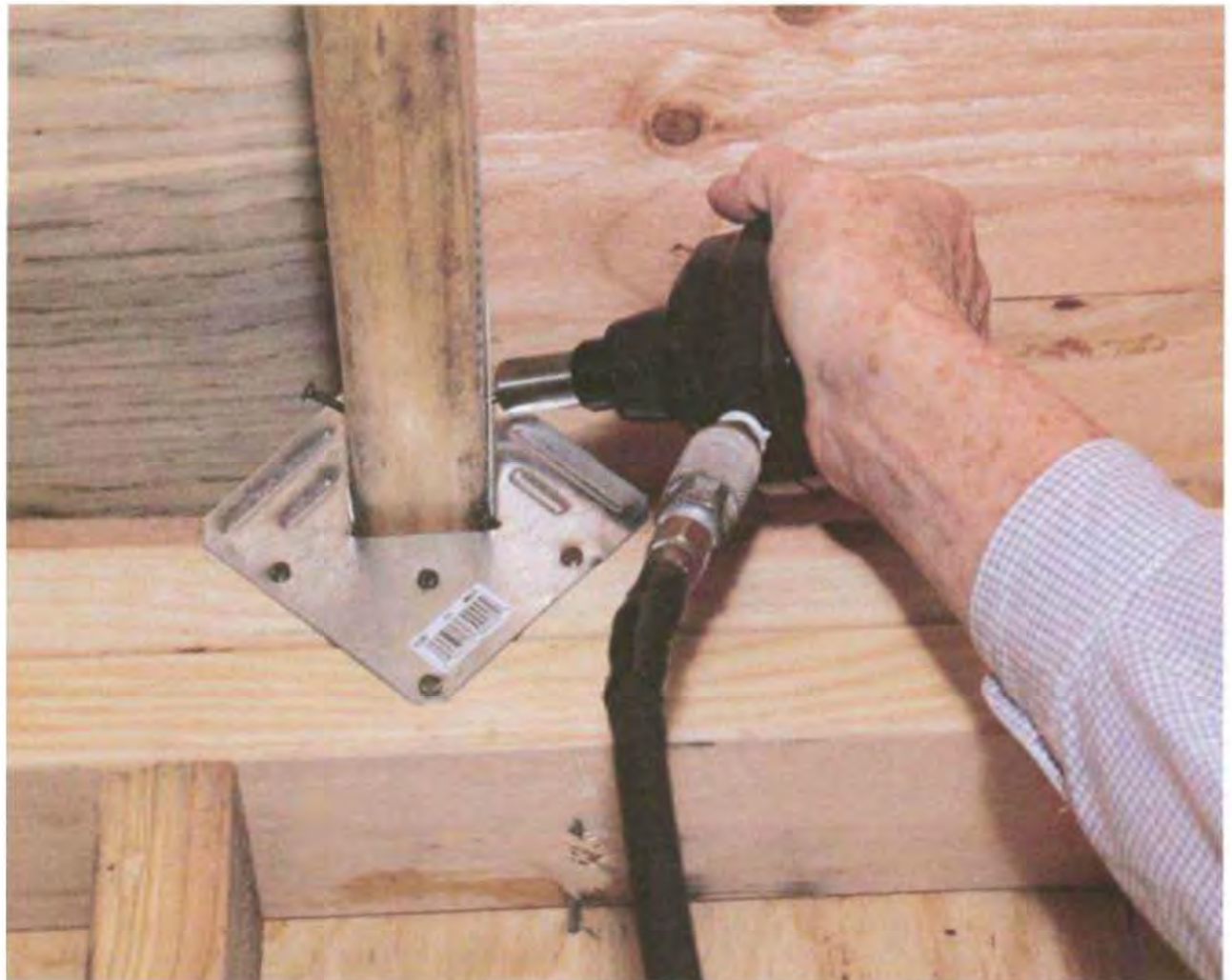
A palm nailer can drive nails in tight places, as when installing a joist hanger. (Photo by Roe A. Osborn.)
