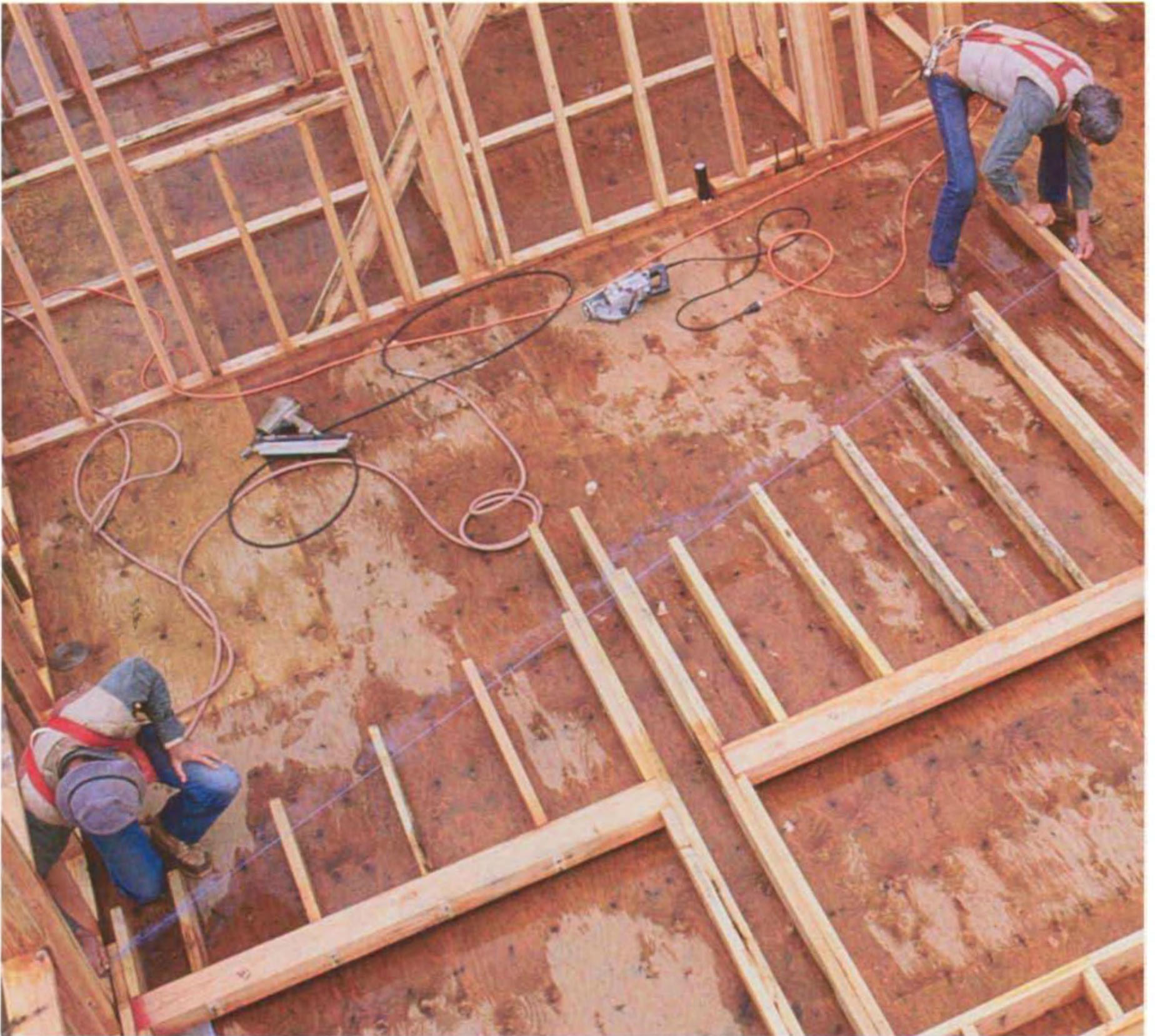
Once walls are laid out and plated, they are assembled piece by piece on the floor. Sometimes the studs are marked and cut to length in place. (Photo by Roger Turk.)
