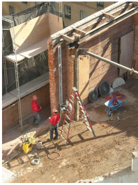
Deconstructing a building to save some components is much more complex than demolishing an entire structure.
