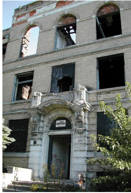
As buildings age, they struggle to provide the same level of comfort and enjoyment that well-designed modern buildings can. Not all are worth preserving.
