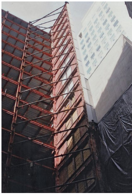
Removal and replacement of structural components generally requires shoring the remaining elements.
