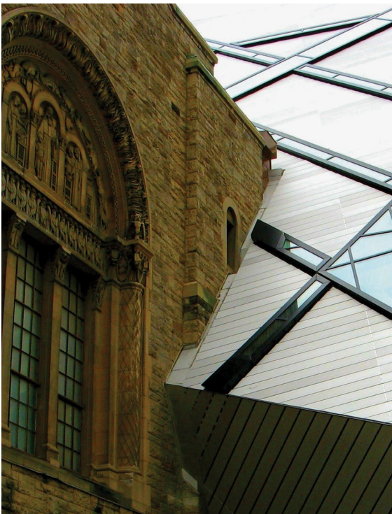
Detailing the intersection of new and old structures can be challenging, especially exterior joints that need to resist environmental forces. Detail of the Royal Ontario Museum, designed by Studio Daniel Libeskind, Ontario, 2007 Photographer: Brother Randy Greve
