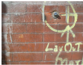
Cleaning the exterior of an existing building can be an involved and expensive process.
