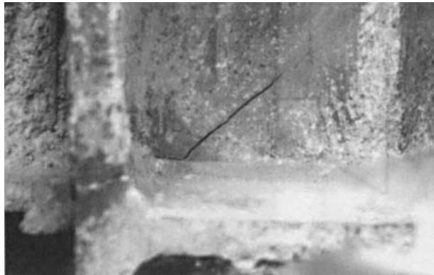
FIGURE 8.10 Photograph of crack through the column flange and into the column web or panel zone of connection.
