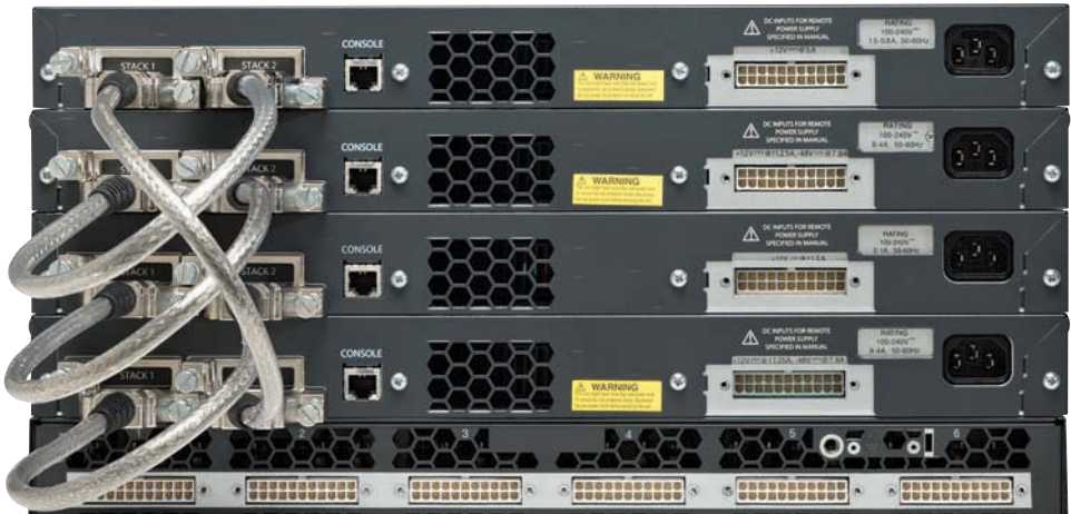
Figure 11-9 Cisco Catalyst 3750 Switch Stack
