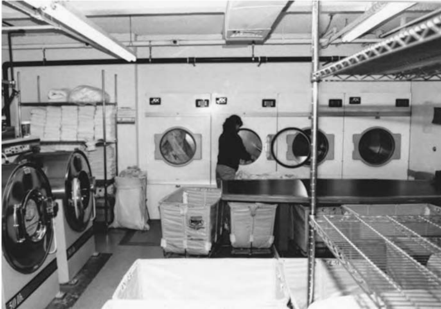
Figure 15-38 Laundry layout indicating how linen flows from washer to dryer to folding tables. Laundry hampers are rolled under folding table with cleaned and dried linen to be folded. (Photo taken with permission.)
