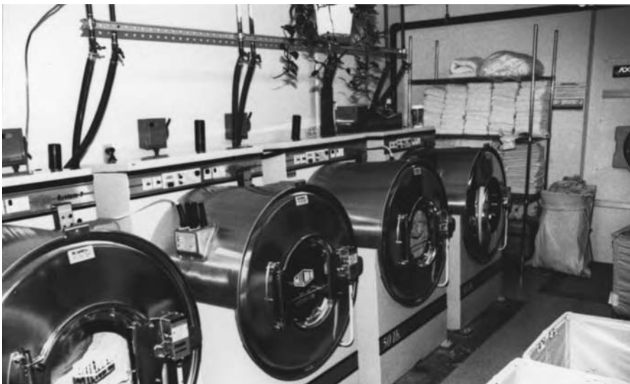
Figure 15-24 A bank of four 50-pound washers plumbed for automatic chemical and water intake. (Photo taken with permission.)
