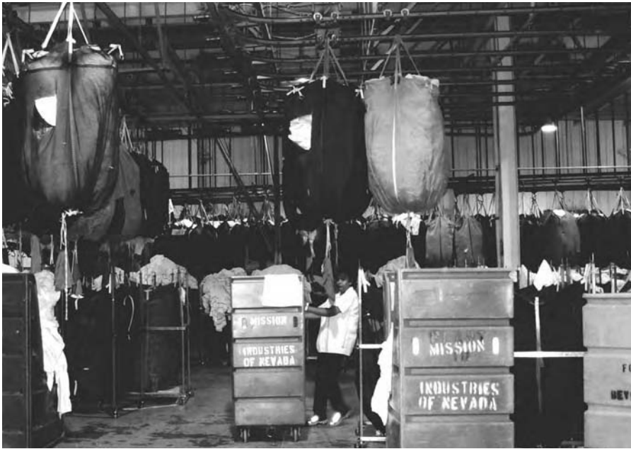
Figure 15-15 Some of the linen is not shot through tubes, but moved in giant laundry bags on an overhead conveyor system. The linen is emptied by releasing a drawstring on the bottom. (Photograph courtesy of Mission Industries, Las Vegas.)
