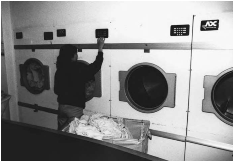
Figure 15-25 Four 100-pound dryers make a compatible arrangement with four 50-lb. washers. (Photo taken with permission.)
