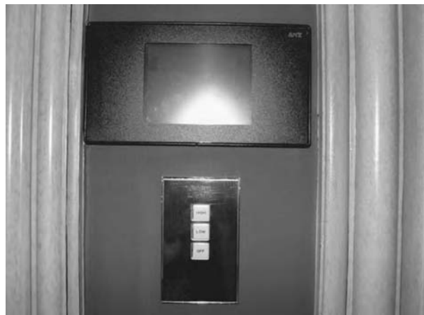
Figure 4-10 In the Villa Suites at Bellagio, a state-of-the-art communication and control system has been installed for the guest's convenience. It can do everything from opening the drapes to summoning the butler. These touch pads are conveniently located throughout the suite, from the night table, as shown in the first photo, to the wall of the dining room shown in the second photograph. (Photos courtesy of Bellagio, MGM Mirage, Las Vegas, Nevada.)
