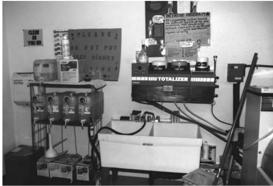
Figure 15-27 Soak sink and chemical mixing center. Note detergent lines leading to washing machines. Other chemicals are arranged for proper dispensing. Soak sink is an important item on laundry small equipment list. (Photo taken with permission.)
