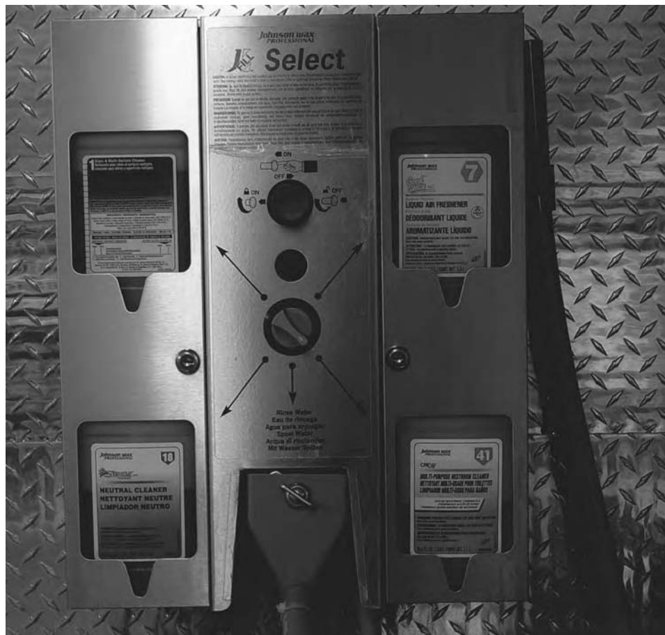
Figure 6-9 A close-up of a chemical mixing station in a satellite linen and storage room. (Courtesy of Bellagio MGM Mirage, Las Vegas, Nevada.)
